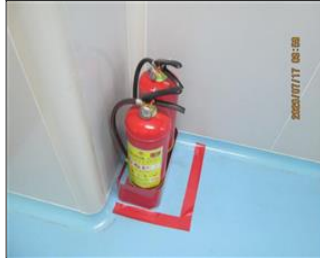
Photo of fire safety equipment fire extinguishers.JPG
