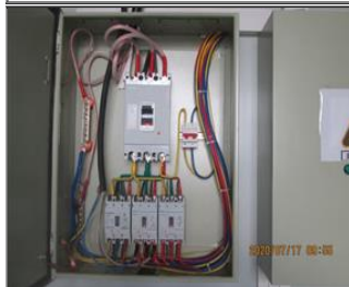
Photo of non-conformity NC The electrical box was not locked for protection and partial electrical parts were exposed.JPG
