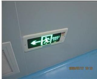
Photo of fire safety equipment evacuation sign.JPG
