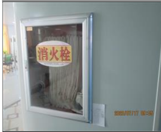
Photo of fire safety equipment fire hydrant.JPG
