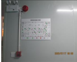
Photo of fire safety equipment fire alarm.JPG
