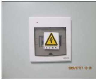
Photo of fire safety equipment electric facility.JPG
